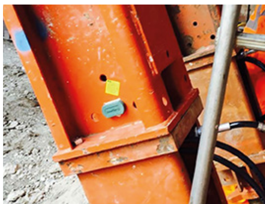
Figure 11 Wireless sensor network (WSN) system pad on a girder
