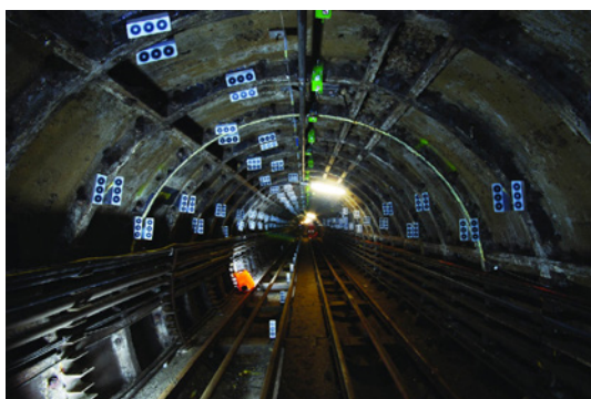
Figure 10 Fibre optic (FO) sensors pads for monitoring a tunnel
