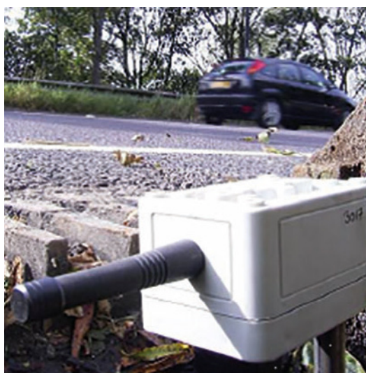
Figure 17 Self-Monitoring Drainage Gully
