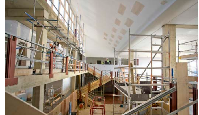
The first floor will accommodate office space for staff and research students arranged around the courtyard, together with additional meeting and seminar rooms, all reached via the the main stairs in the atrium and adjacent to the open Common Room.
